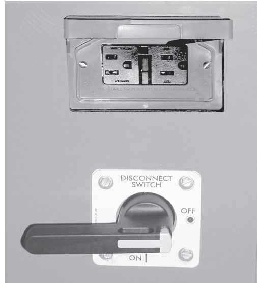
Figure 3: Convenience Outlet/Disconnect Switch
