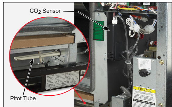
Figure 40: CO2 Sensor For Demand Control Ventilation
