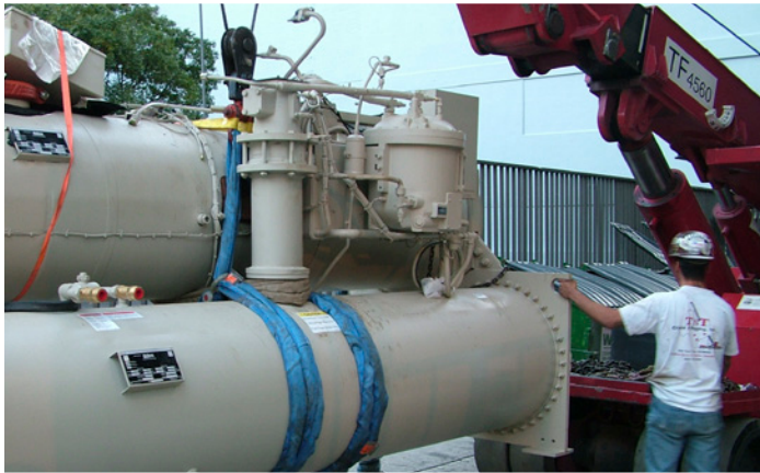
The new Daikin centrifugal chiller arrives partially disassembled for installation in the ground floor of the 823 Congress building.
