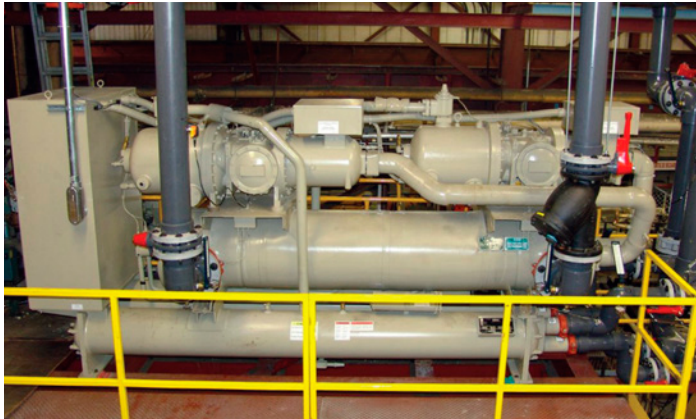
The Daikin water-cooled screw compressor Model WGS Chiller installed at the Camoplast automotive component injection molding facility is part of the energy award winning system that reduced annual energy costs by 70%.
