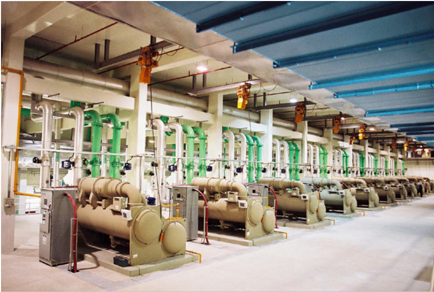
Daikin chillers in the central plant
