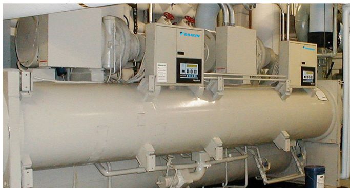
The Magnitude chiller was installed next to an older screw compressor chiller and the new chiller is dramatically quieter than the other machine.
