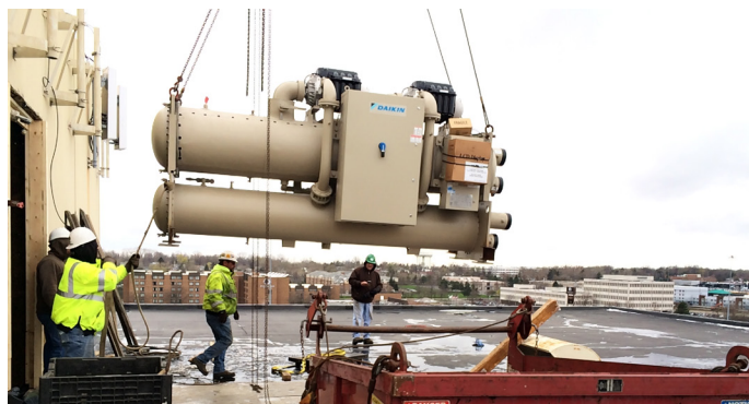
The new Daikin chiller is lifted onto the Orange Place building for installation in the penthouse mechanical room.
