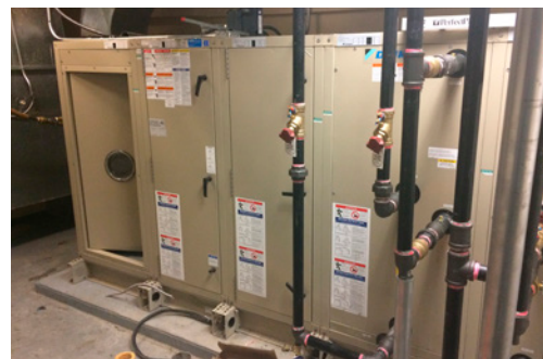
Dawson Creek Campus equipment room
