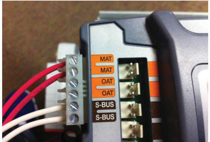
Figure 18: Jade Control Connections
