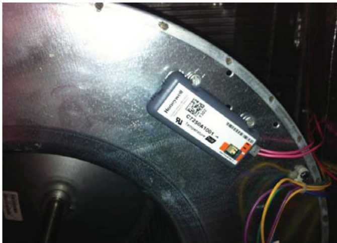
Figure 28: Attached Mixed Air Sensor on Blower
