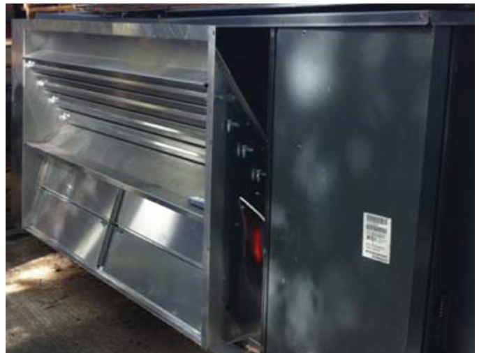
Figure 22: Evaporator Support Brackets
