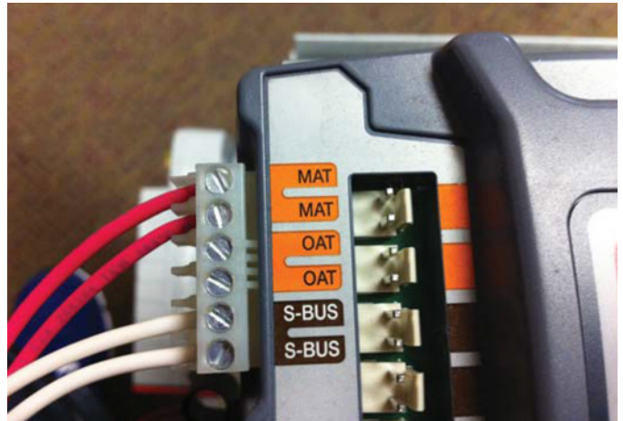
Figure 10: Jade Control Connections
