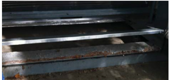
Figure 21: Evaporator Opening Side Posts
