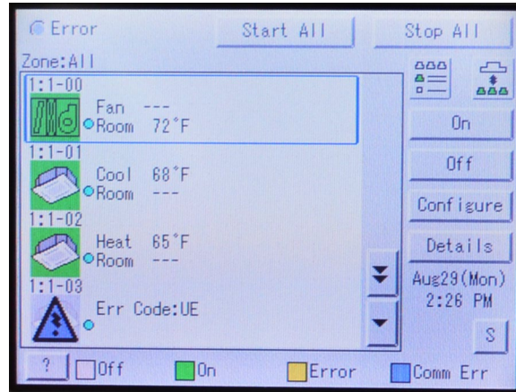
Figure 24, Air Handler in Unoccupied Operation
