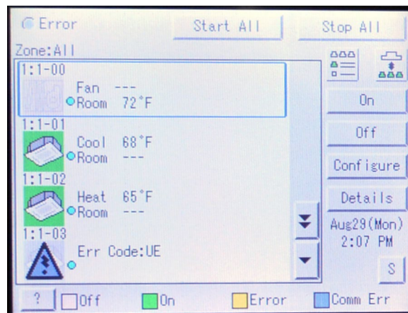
Figure 23, Air Handler Unit in Unoccupied Mode
