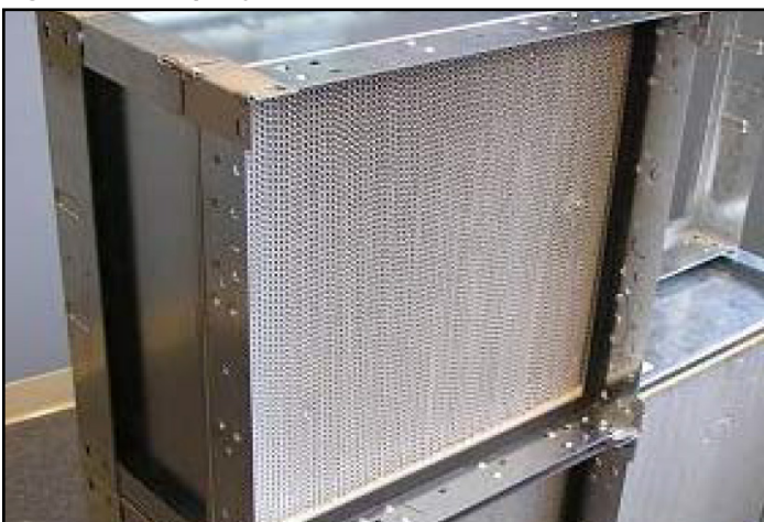
Figure 133: Properly Installed HEPA Filter
