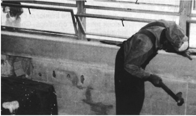
Figure 13: The Interior Wall is Knocked Out in the Area Cut for the Wall Sleeve
