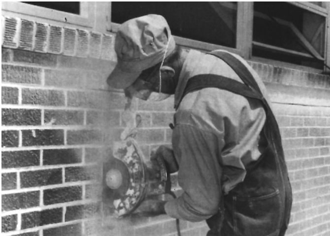
Figure 10: Cutting the Outside Wall Rough Opening Slightly Larger Than the Size of the Louver
