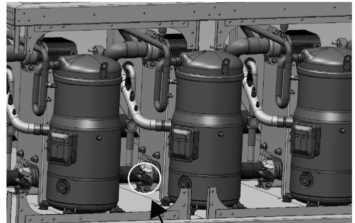
Figure 33: Condenser Water Supply Drain Valve
