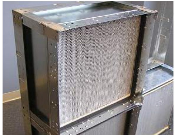
Figure 34: Properly Installed HEPA Filter
