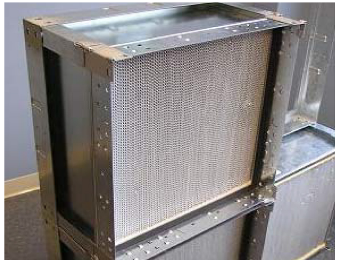
Figure 34: Properly Installed HEPA Filter
