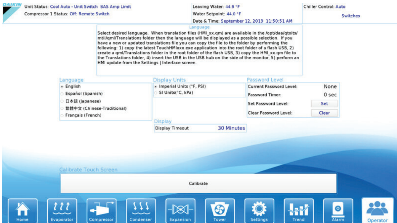
Figure 37: Operator View Screen
