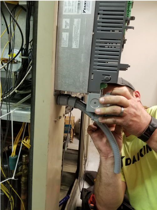
Figure 12: Actuators for Waterside Economizer
