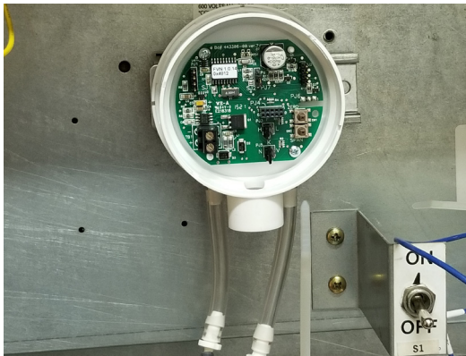
Figure 9: Duct Static Pressure (DSP) Transducer
