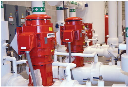
Figure 2.1 Pumps for a Central Chiller Plant
