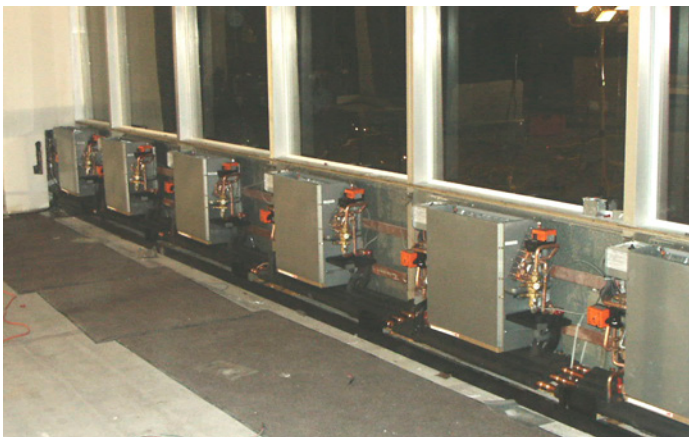
Factory-installed piping connected one unit to the next using a solderless coupling technology.
