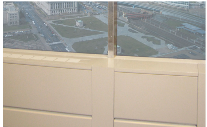
Custom-designed fan coil housings provide a fresh look to each office and frame the skyscraper view of downtown Cleveland.
