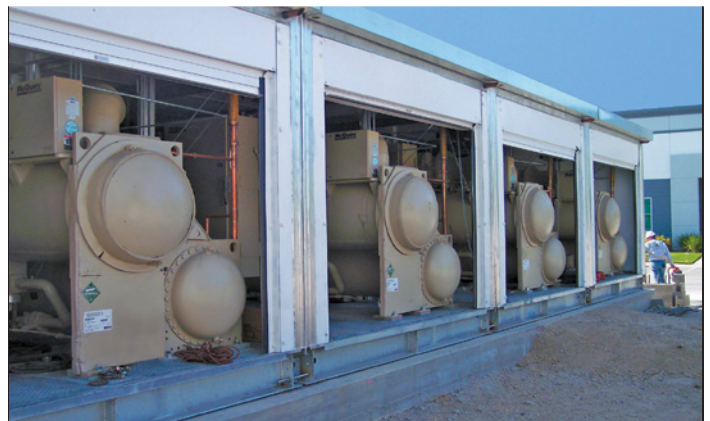
Four of the six Daikin Modular Central Plants that provide mission critical cooling for the Herakles Data Center.
