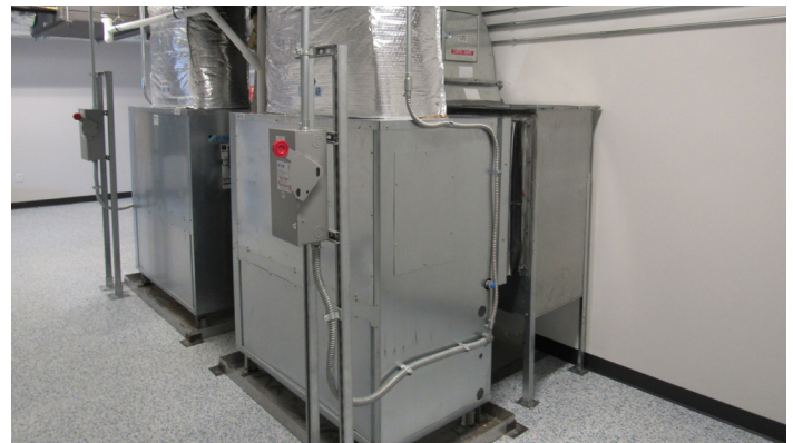
Two large capacity WSHPs with hot gas reheat provided solutions for VIP's data center space requirements.
