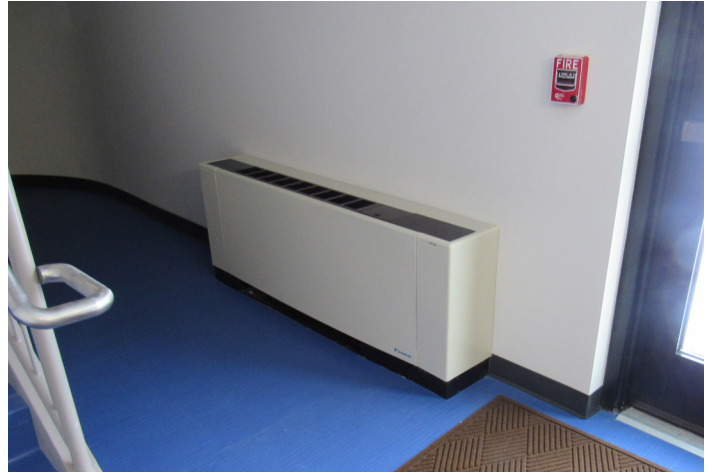
VIP also incorporated Daikin Enfinity console WSHPs for supplemental heating and cooling in specific areas in the new building.
