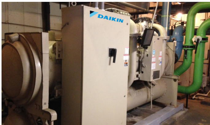
Daikin Magnitude chillers contribute to impressive energy savings.
