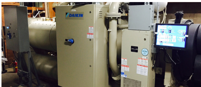
Up and running, the energy efficient Magnitude chiller is expected to save approximately $50,000 per year in energy costs.
