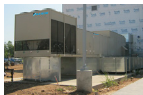
Daikin 79-ton RoofPak
